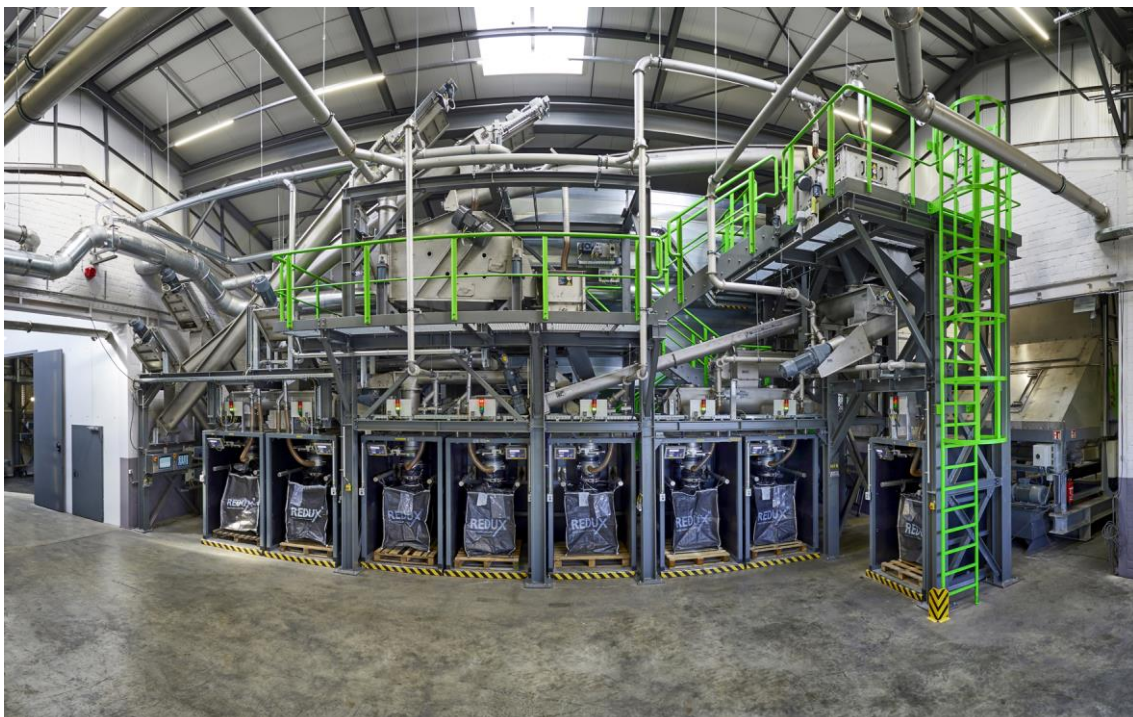
Recycling plant for Lithium-Ion Batteries in Bremerhaven, photo credit: Saubermacher
